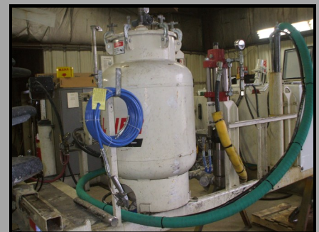
Pressurized Bead Tank
