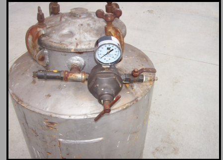
Regulator and new pressure gauge
