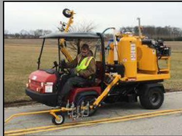
Maintains traffic flow, 10' turning radius
